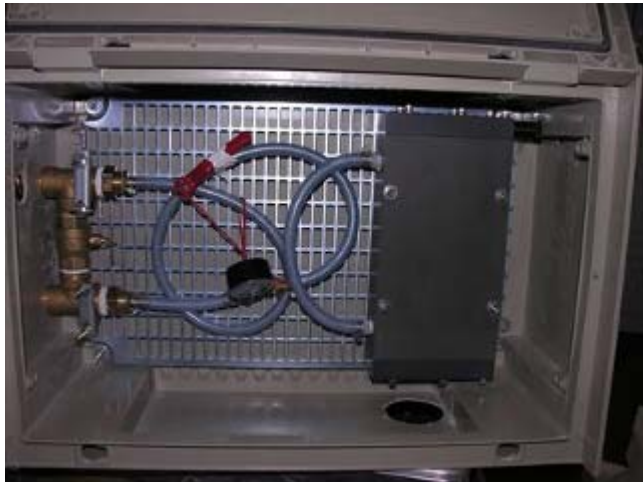
SBE45 bypassed for tests
